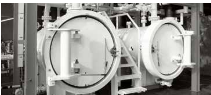
Pipe and boiler thermal insulating coating
