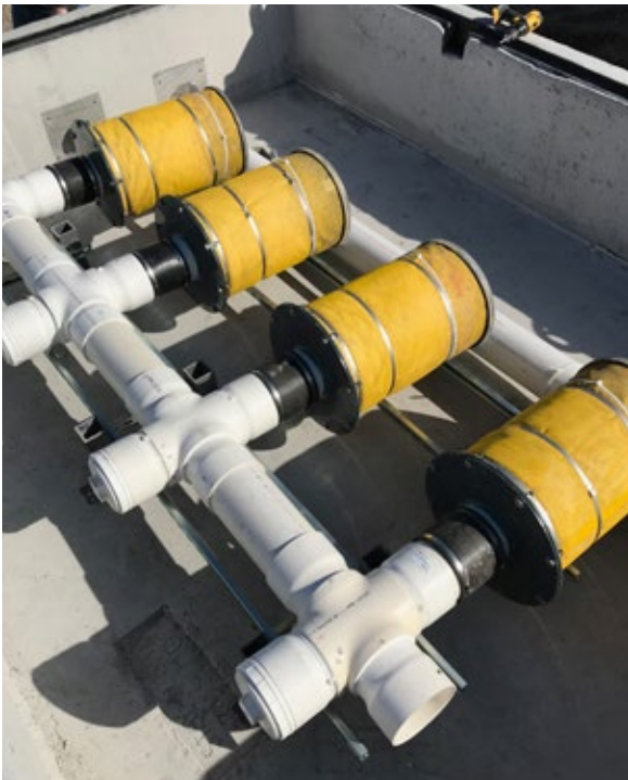
Multi-port HFF in vault
