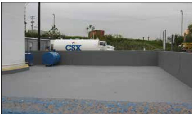
Diesel fuel containment
