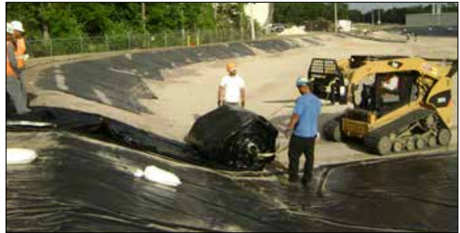
Approximately one foot of dirt was removed and elevation was established for storm water drainage.
