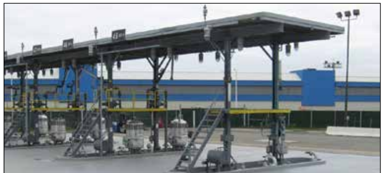
Truck loading rack
