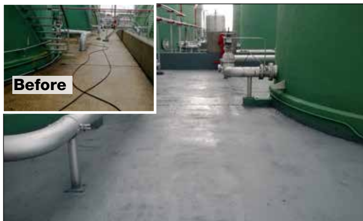
JFK airport jet fuel tank farm concrete containment coating
