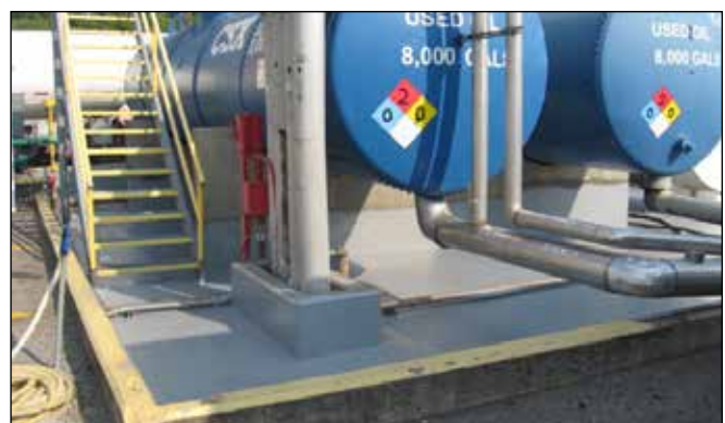
Fuel containment area
